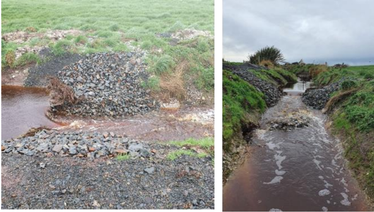
Figure 16: Site 3 after second failure (10 September 2021).
