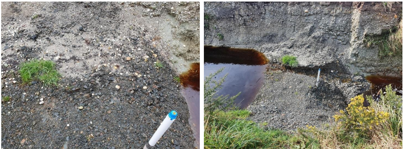
Figure 12: Site 1 Gravel weir partial erosion (left) and subsequent initial failure (right), July 2021.
