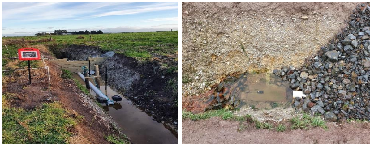
Figure 10: Site 5 wooden weir following installation looking downstream (left) and flow monitoring equipment installed downstream of culvert pipe (right).
