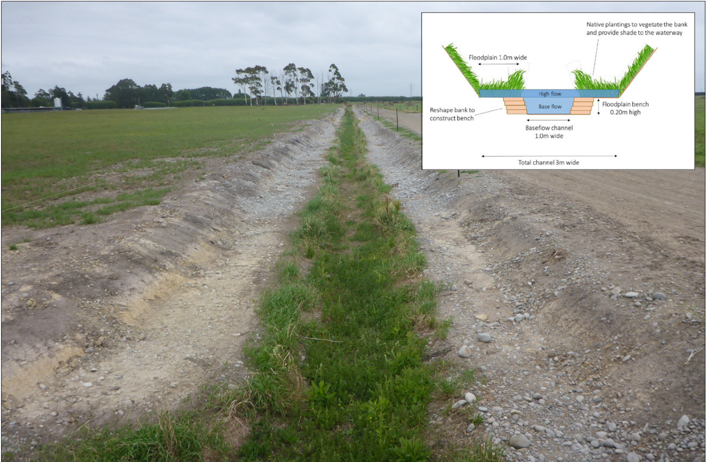
Figure 11. Bioreactor (A) before and (B) after construction the two stage channel began. The height of the benches was determined from the stage height hydrographs.
